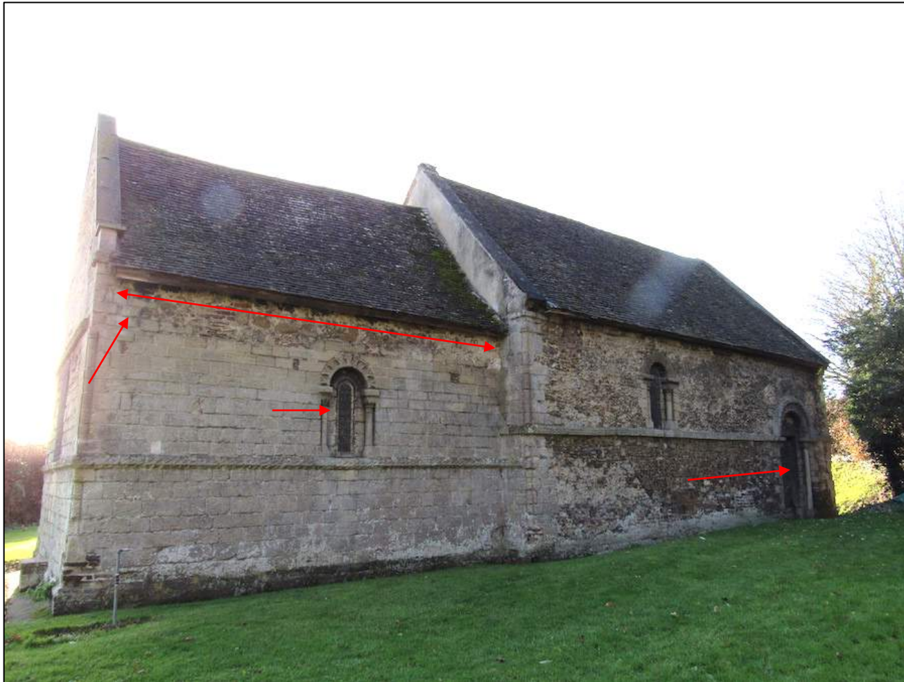
Figure 25: Photograph of the Cambridge Leper Chapel looking south. The red arrow at the top of the chancel shows a substantial repair and the introduction of new rubblestone and brick materials near the roofline. The red arrow at the far left in the chancel illustrates a 12 th century worked stone that was salvaged and used in the rebuilding of the wall. The red arrow pointing to the chancel window shows work that was completed on the window in the 15 th century. In the nave, the arrow at the right shows the door that has been bricked-in (Gjesfjeld 2019).
