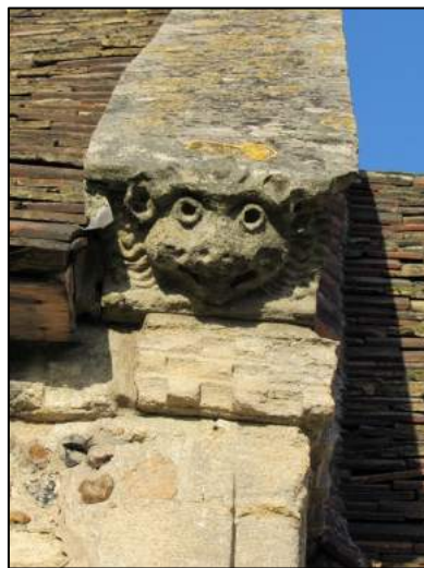
Figures 20 and 21: Photograph at the left illustrates detail of one of the grotesque figures on the nave. The bottom right photo shows the nave window on the south facade of the building. The red arrows show a repair to the left shaft as well as the introduction of a replacement shaft on the right (Gjesfjeld 2019).
